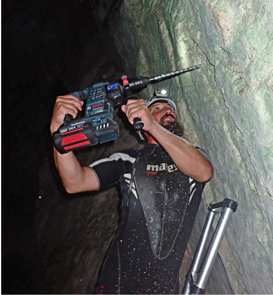
Figure 4-21. Instalment of the mount of an infrared camera system in Zakynthos
